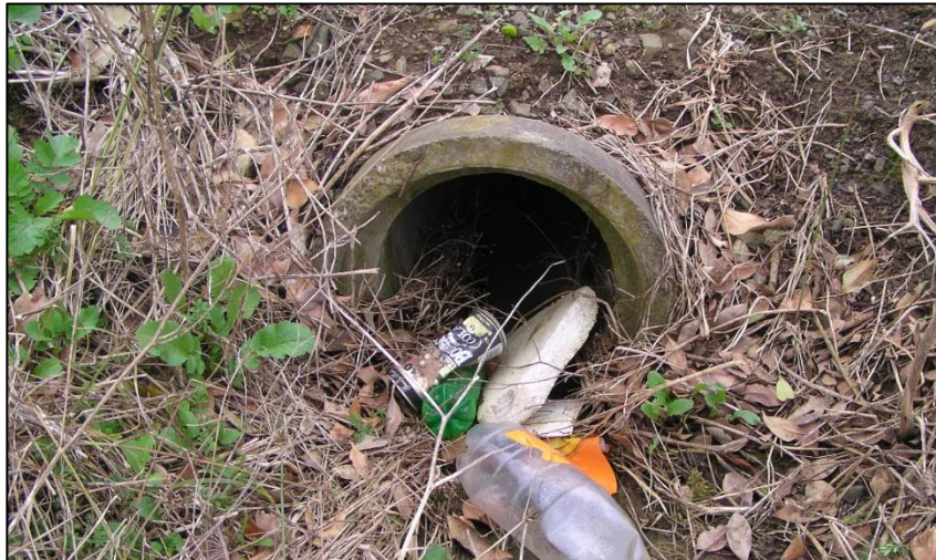
Undersized entrance culvert that will not cope with a "large" storm.
