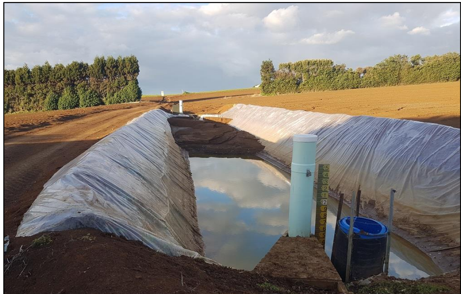
Bedload accumulating at the entrance to the SRP, showing just how quickly bedload drops out when the flow is slowed.
