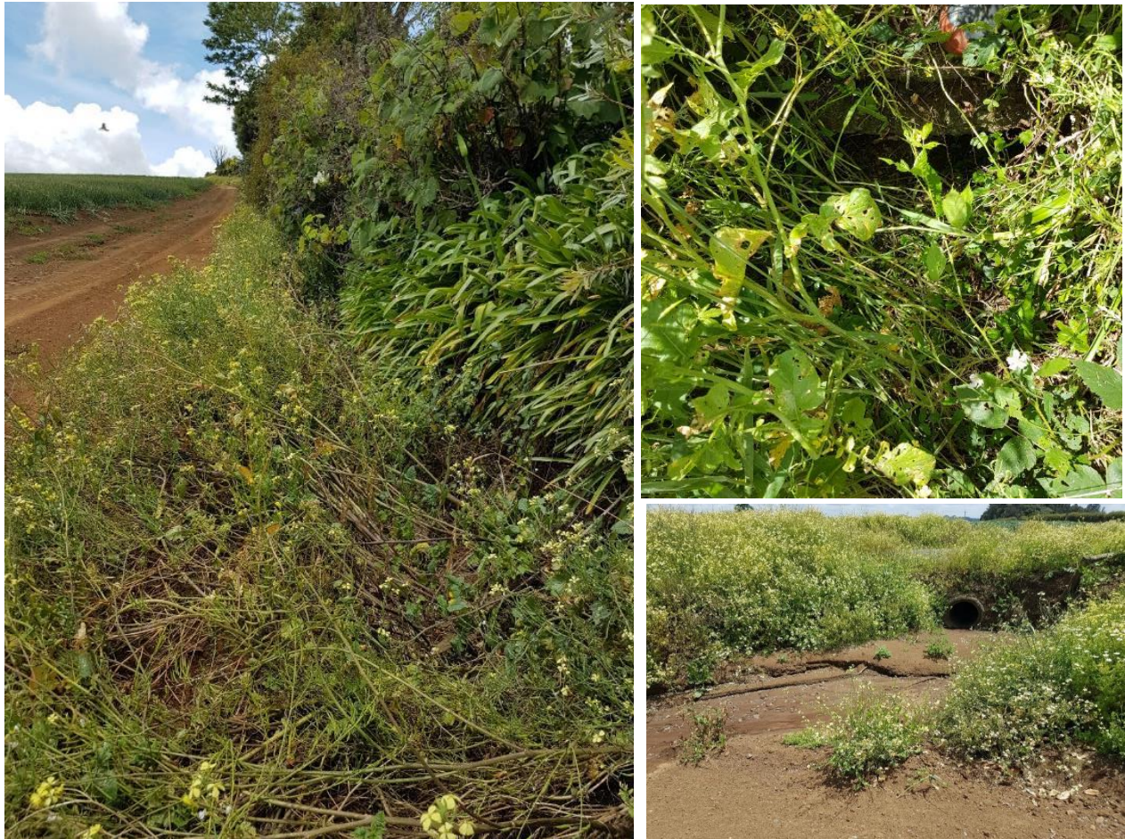
Figure 7. From top left clockwise: i) Overgrown and shallow interception drain along southern boundary. ii) Blocked culvert from southern boundary interception drain. iii) Culvert leading to SRP2.
