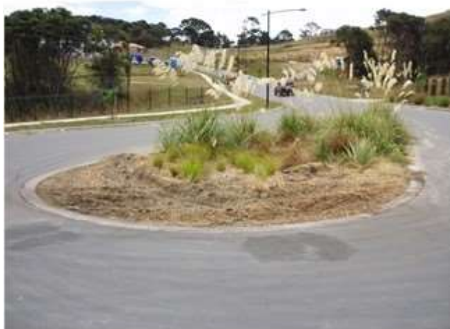
Raingarden with inappropriate traffic crossings
