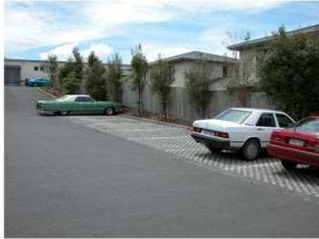
Permeable paving on a library parking lot
