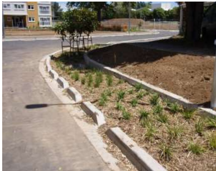
Bioretention construction - sediment entry is compromising future performance
