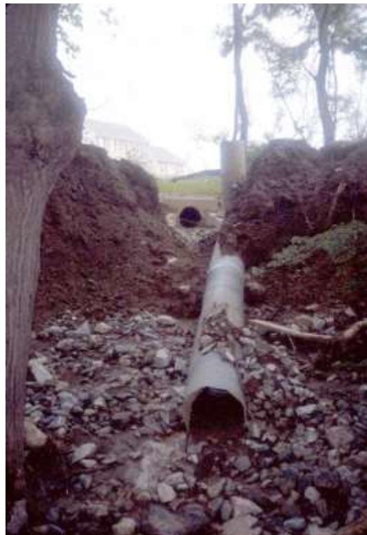
Pond failure resulting from lack of anti-seep collars around outlet pipe
