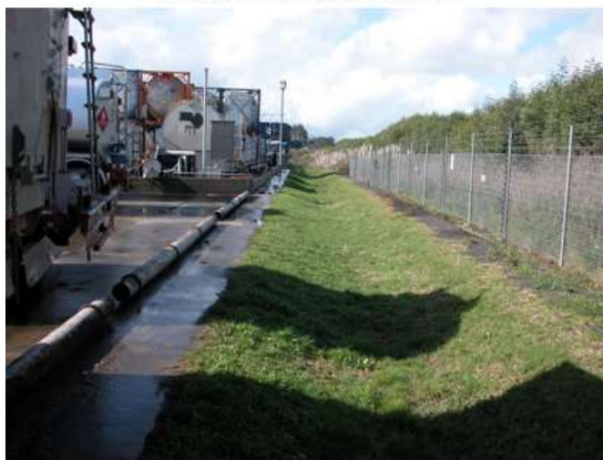
Swale providing pre-treatment of industrial runoff prior to runoff entering a sand filter
