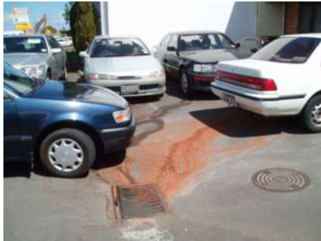
Staining that indicates discharge of contaminants into the stormwater system
