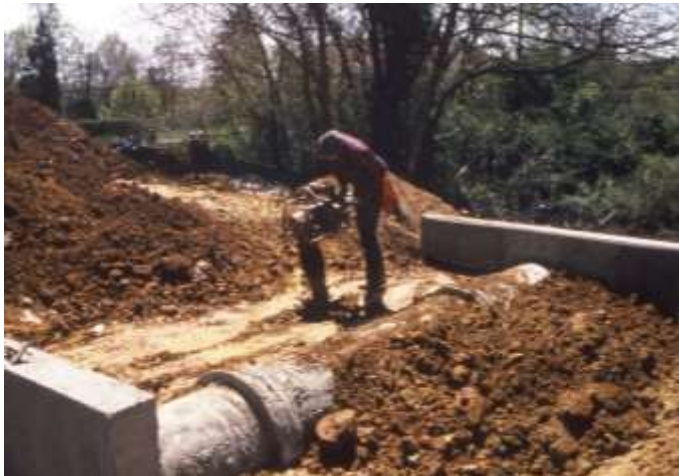
Vibratory compactor being used to compact material around the outlet pipe with anti-seep collar
