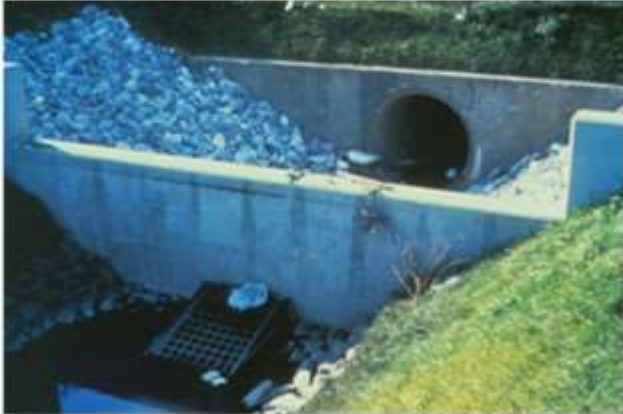
Retrofit of a culvert with extended detention for stream channel erosion reduction and some water quality benefit
