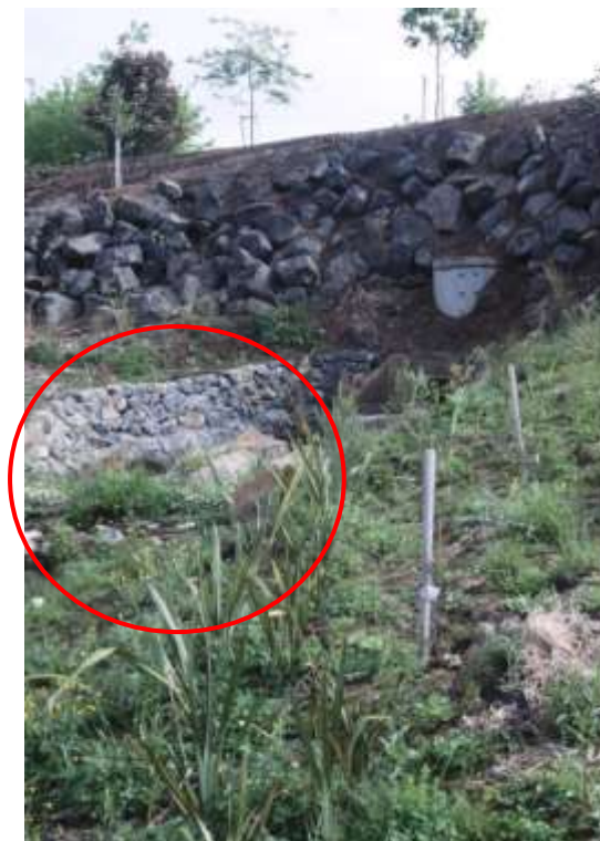
Sediment forebay clogged with sediment and needing to be cleaned out
