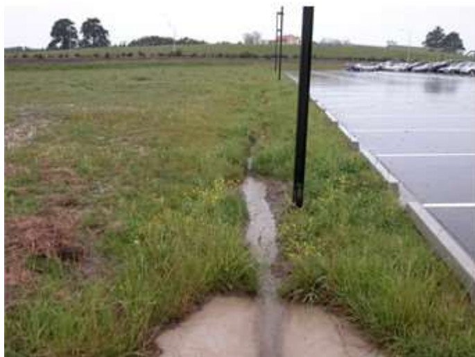
Concentrated flow in a swale causing erosion
