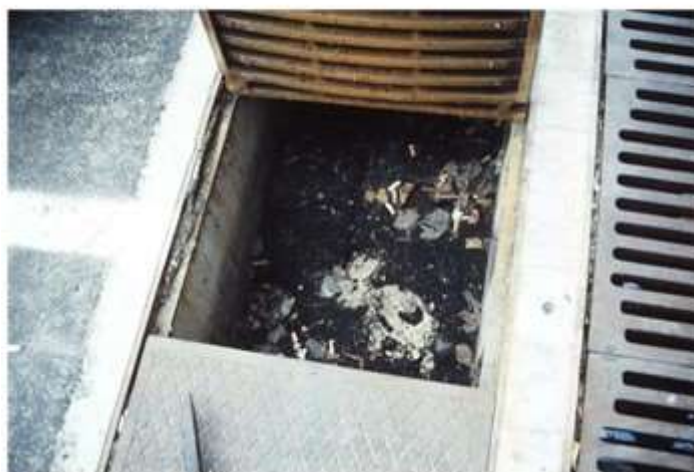
Sand filter clogged by oil and grease
