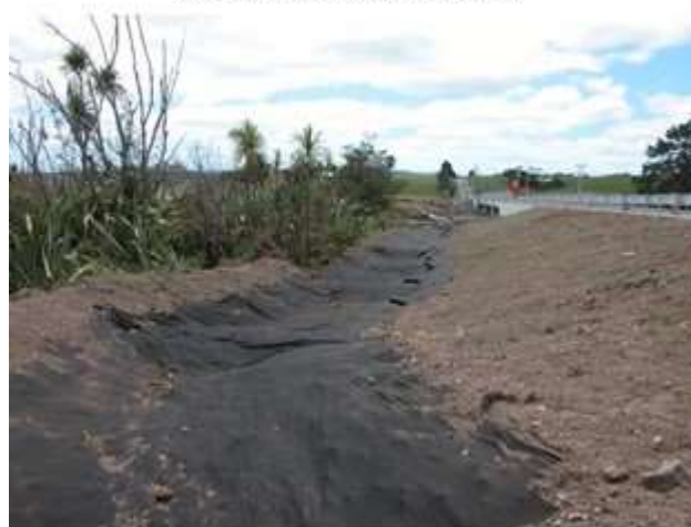
Wetland swale showing check dams prior to placement of soil and plants
