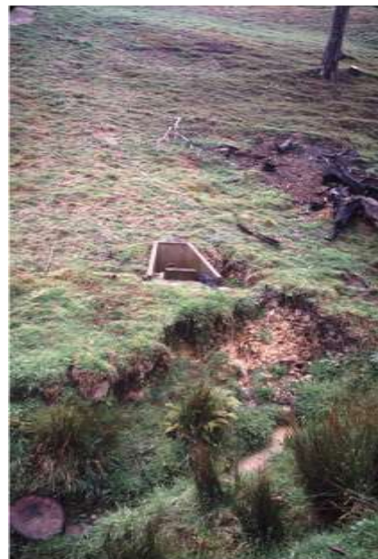
Example of erosion at a pipe outfall
