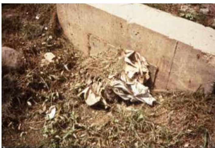
Extended detention outlet clogged and in need of maintenance
