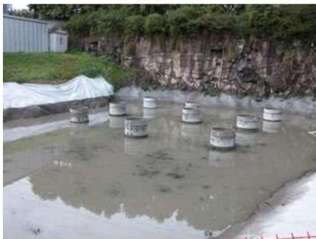
Infiltration of runoff from an industrial site after treatment using a sand filter
