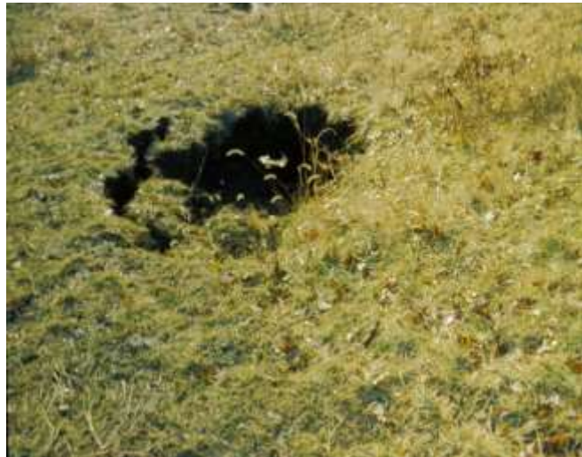
Downstream side of a stormwater pond embankment where piping of flow is causing dam failure
