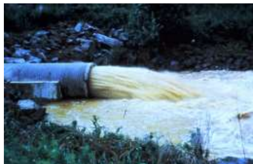
Stormwater discharge into a stream
