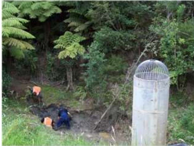
Stormwater pond being maintained by having the silt sucked out by vacuuming
