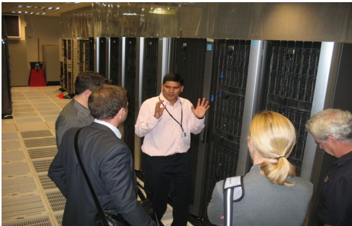
Figure 32: Racks of experimental servers, set up to determine upper operating temperature limits. HP Labs Palo Alto.
