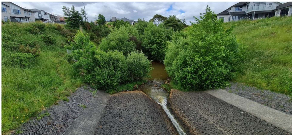
Photograph 1: Vegetation observed around the stilling basin downstream of Magellan Lake showing grey willow growing around the stilling basin.
