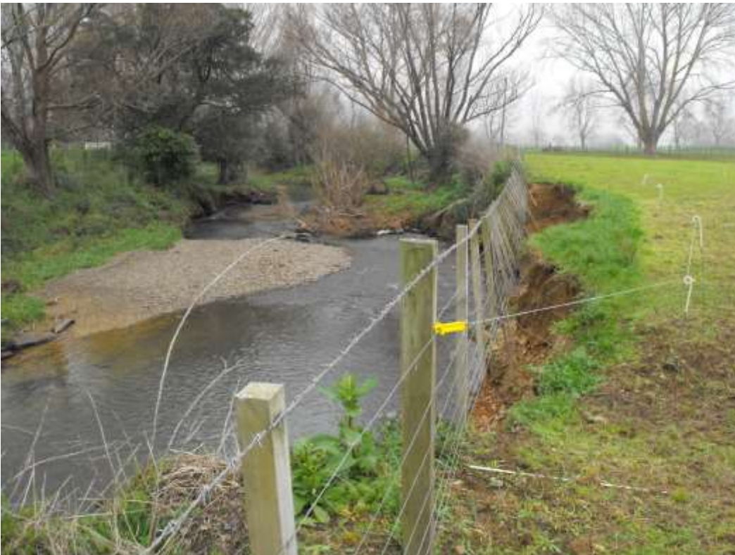
Erosion along the Mangawara Stream.
