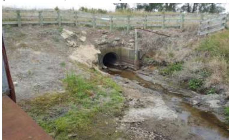
Figure 2: Inlet of gravity flow outlet pipe at Okowhao Pump Station, February 2017. Photo: Taroi Rawiri, Waahi Whaanui
