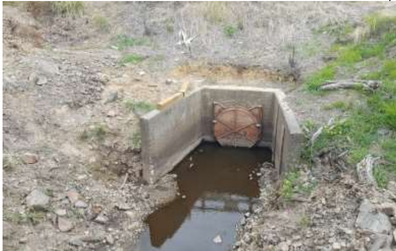
Figure 3: Outlet of gravity flow outlet pipe Okowhao Pump Station. Photo: Taroi Rawiri, Waahi Whaanui
