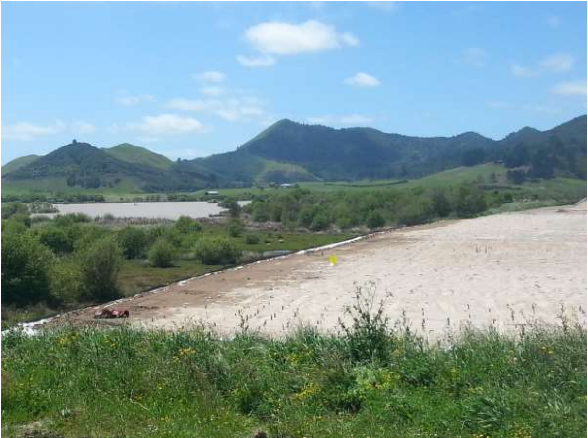
Waikato Expressway under construction along the southern margin of Lake Kimihia. The hills in the background are part of the Lake Kimihia catchment.
