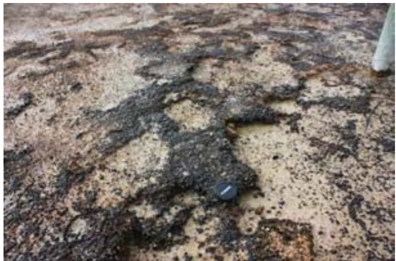
Plates 77 and 78: Deteriorating Sinter Terrace. Structure still visible but very brittle/soft underfoot at Feature 1, Wharepapa Road.
