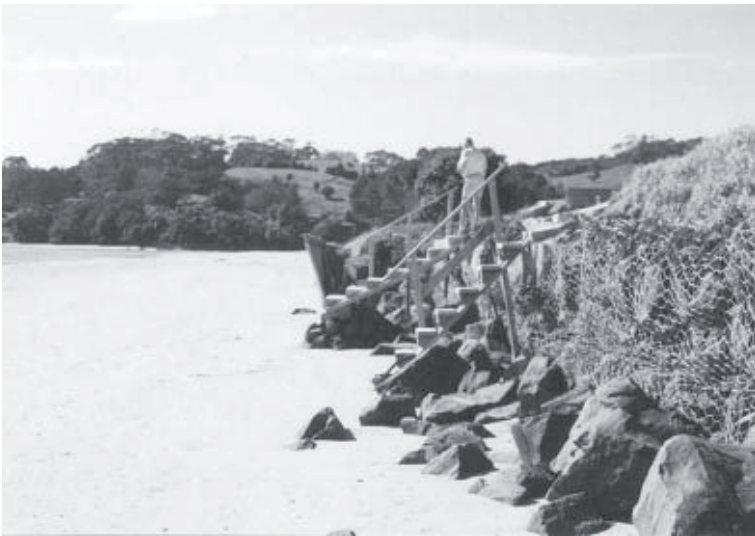
Figure 5: Coastal structures at Cooks Beach, 2001. The structures degrade the appearance of the beach, and the beach level has dropped in front of the structure, restricting public access to and along the beach.
